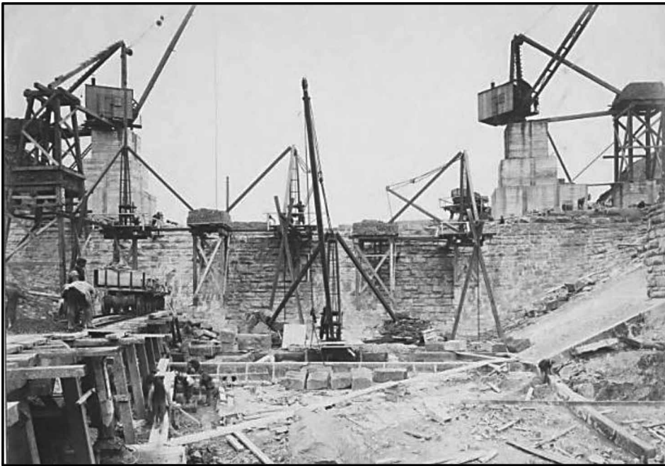
Figure 6 Craig-Goch dam (downstream face) showing reliance on cranes during construction. ©Crown copyright: RCAHMW
