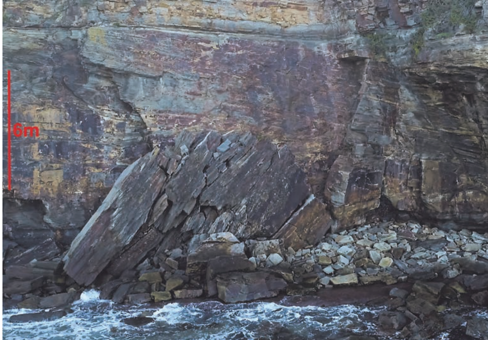
Figure 35. Rotated slab fall on Turimetta Head, initiated by a storm in 2015 and still falling in 2022.
