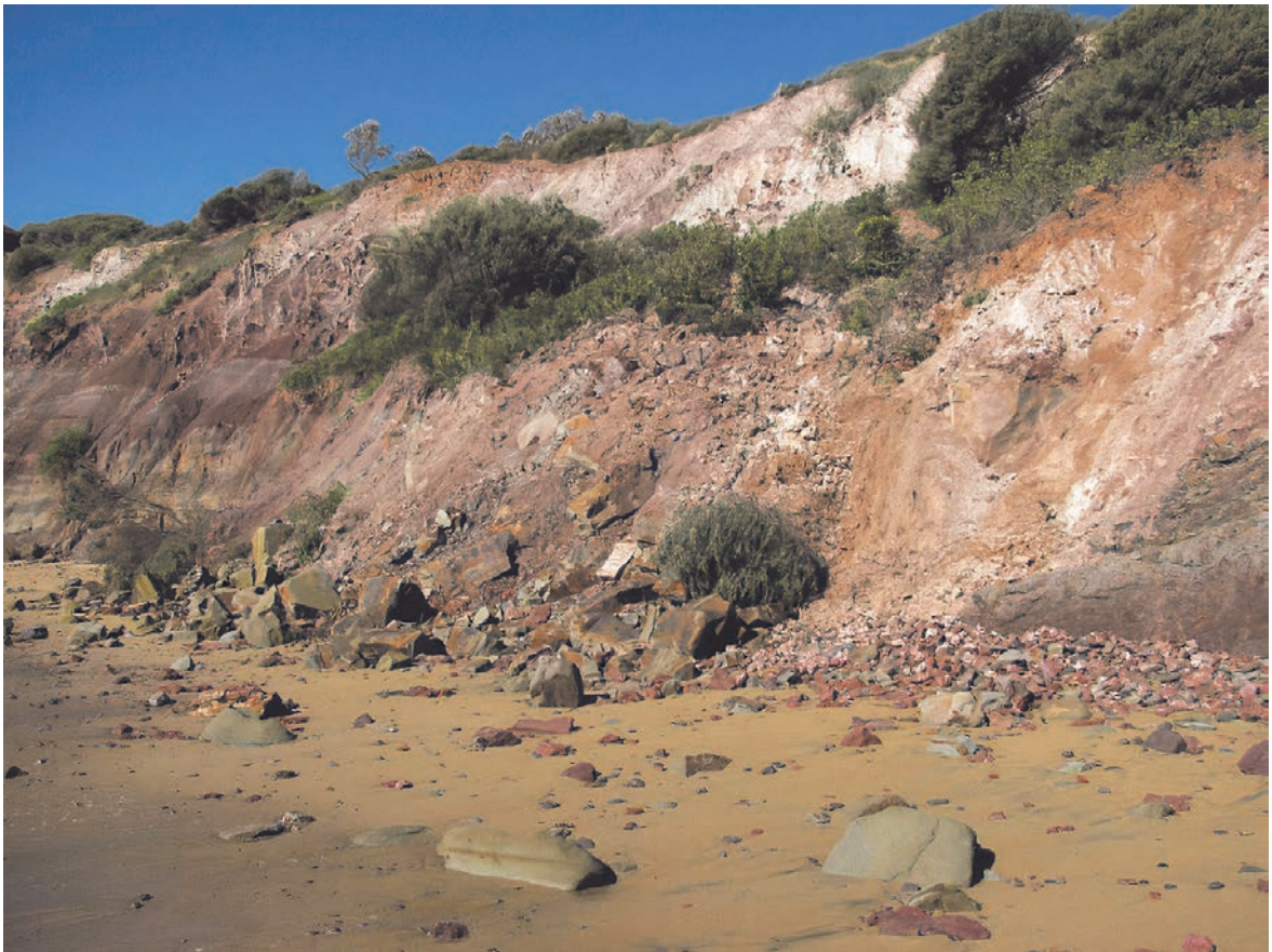
Figure 34. Planar slump in weathered Bald Hill Claystone on Long Reef Point. Photo taken shortly after the initial collapse in 2016.
