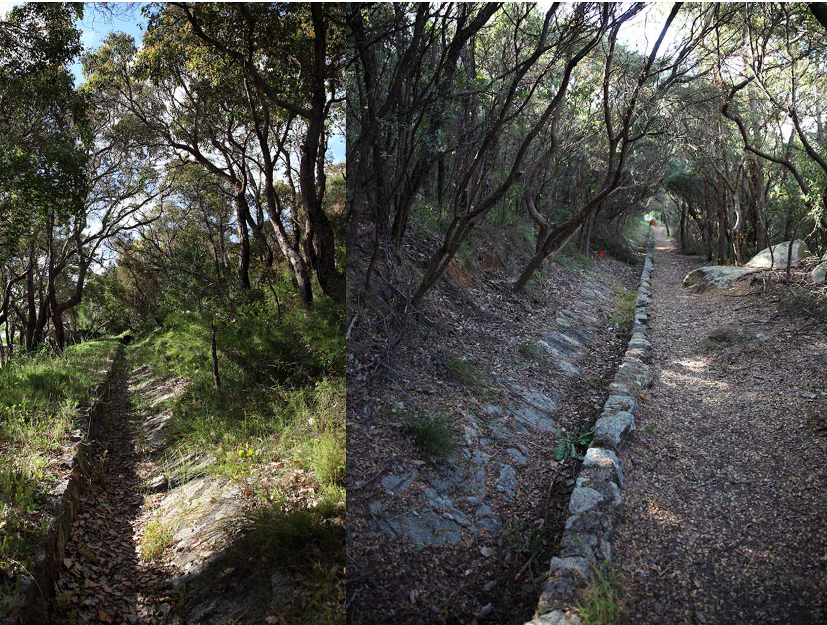
Fig. 3 Mt Clarence interceptor drains constructed 1897–1903. These are close to parallel to the contour and were designed to catch overland flow in the belief that this would stop the town below being flooded. Photos © Perdita Phillips
