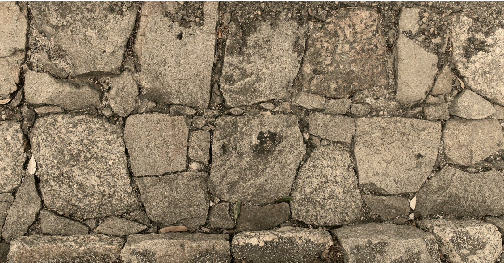
Fig. 7 “Colonial” drains: detail of mortarless construction of kerbing at Duke Street. Strips of bitumen have crumbled, and the permeable pavers have been re-exposed. Water moves across and through . Photo © Perdita Phillips
